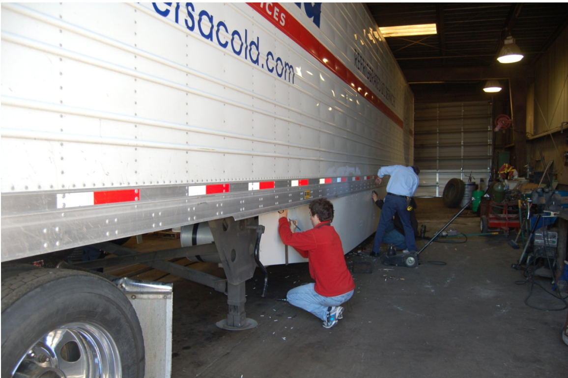
Green Collar workers installing ATDynamics side skirt aerodynamic fairing the morning of the committee meeting
